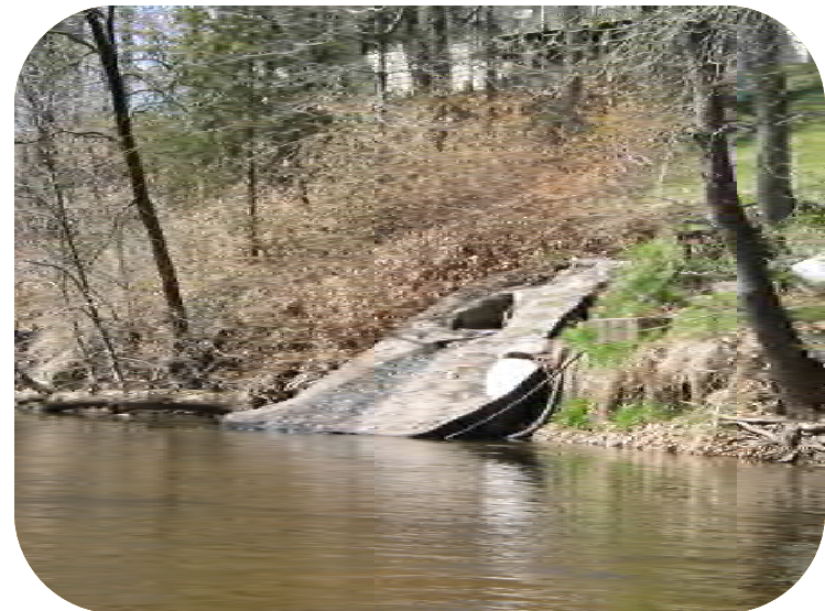
Photo 44 – Approx. 24 in. flared end section exiting bank at midpoint of slope with concrete apron.
