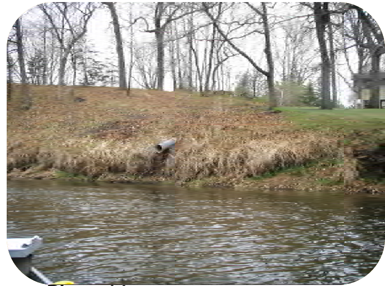
Photo 14 – Overhanging 12" diameter outlet positioned on center of slope.
