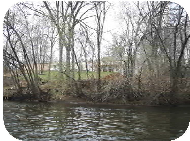
Photo 10 – Cleared all large near-shore trees. Pushed soil over riverbank. Also see photos 11,12, &13.
