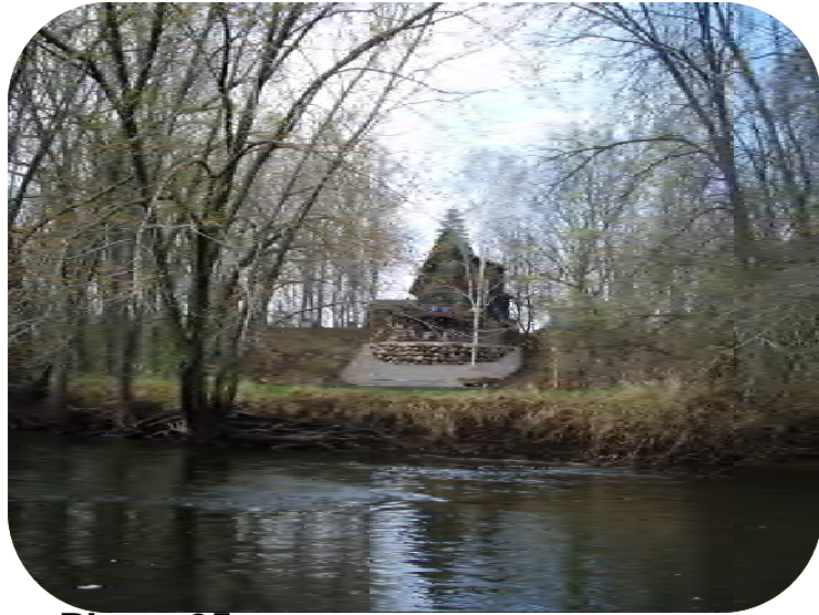
Photo 25 – A-frame house on bluff. Rock work to stabilize toe of slope. Also see Photos 26, 27.
