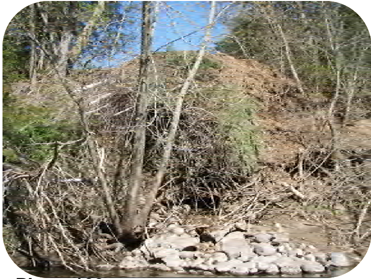
Photo 109 – Approx. 24" flared end section and yard waste piled above. Also see Photos 110, 111, 112, 113.
