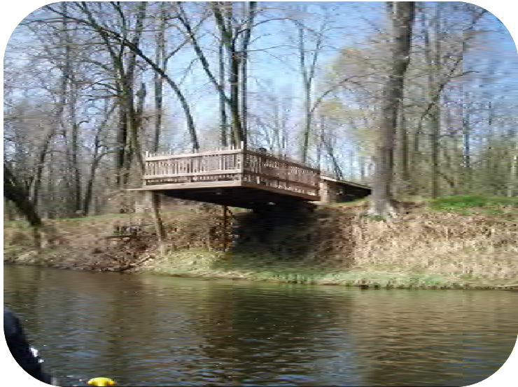
Photo 33 – Approx. 10 ft. by 10 ft. deck cantilevered over water's edge. No apparent erosion.
