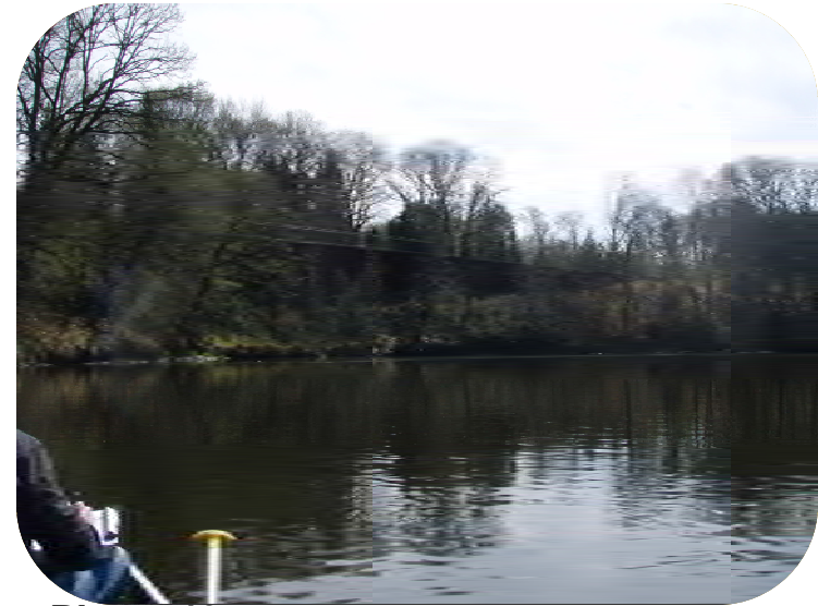
Photo 40 – Driven piling flood wall to eliminate outer bank erosion. Also see Photos 41 and 42.
