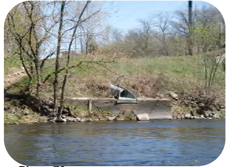
Photo 78 – Viking Blvd. bridge and approx. 18 in. outlet onto concrete slab approx. 4 ft. above water.
