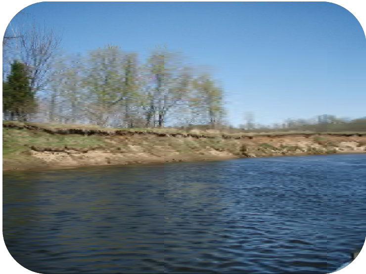
Photo 91 – Severe erosion, 20 ft. back with fence over water. Also see Photos 92, 93, 94, 95, and 96.
