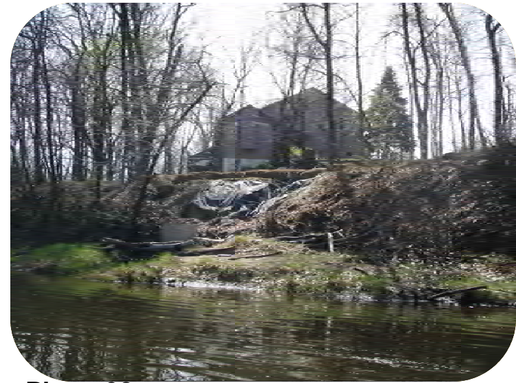
Photo 38 – 12" pipe at toe of bank. Moderate erosion with homeowner-attempted repair. Also see Photo 39.
