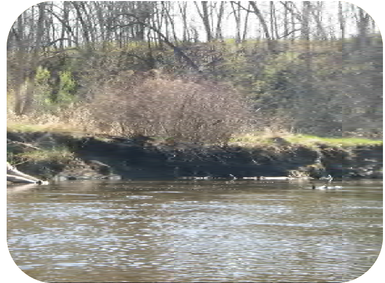
Photo 114 – Moderate erosion. Also see Photo 115.
