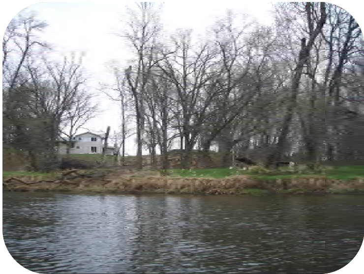
Photo 9 – Earthwork and nearly bare soil (sparse straw cover) associated with home or septic construction.
