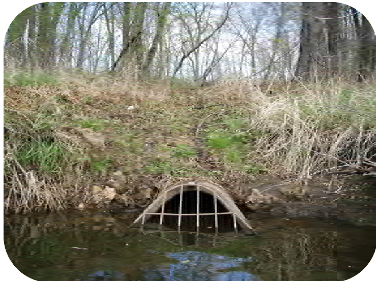
Photo 29 – 36 in. wide, 20 in. tall FES, with trash rack, outlets at water level.
