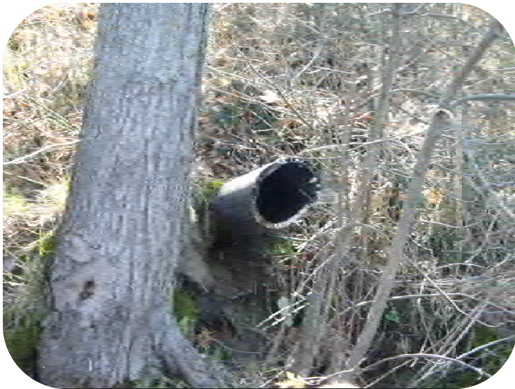
Photo 43 – Outlet, 8 in. plastic pipe exiting lower 1/3 of bank overhanging water. No apparent erosion.
