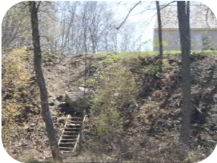
Photo 75 – Erosion along side of stairs leading to water.
