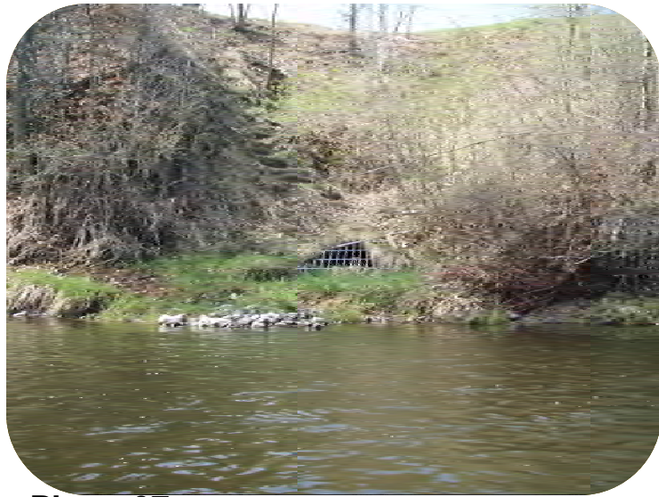
Photo 37 – Outlet with flared end section 66 in. wide, 32 in. tall with trash rack.
