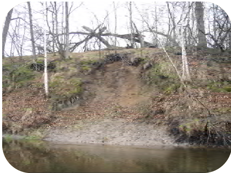
Photo 7 – Outfall pipe high on slope causing bank failure. 6-8" dia pipe.
