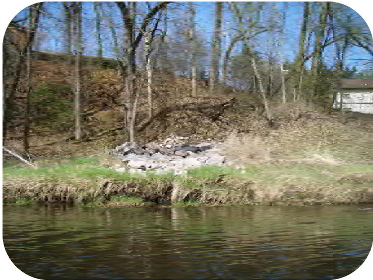
Photo 35 – Outlet 18-24 in diam. with flow separator. Large rock below, no apparent erosion. Also see Photo 36.
