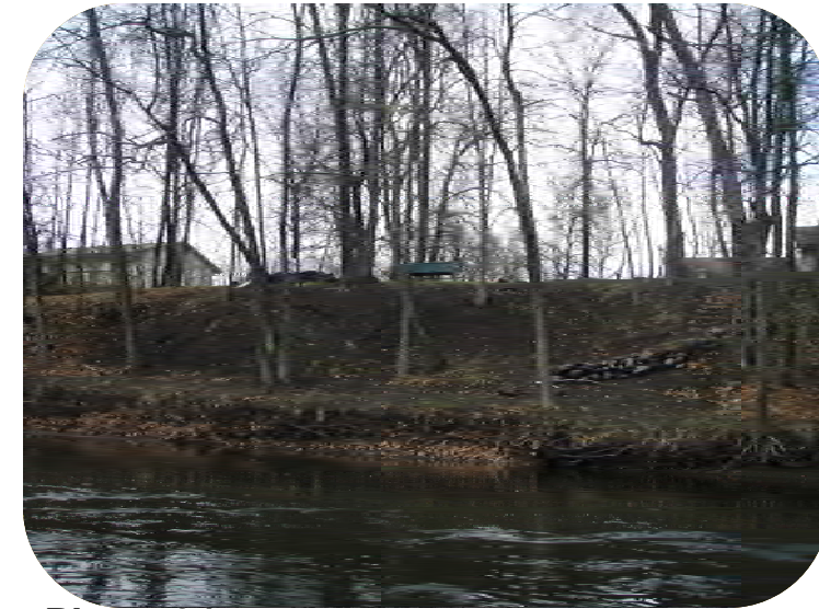
Photo 24 – Removed all ground and leaf cover across slope. No apparent erosion, but a poor practice.
