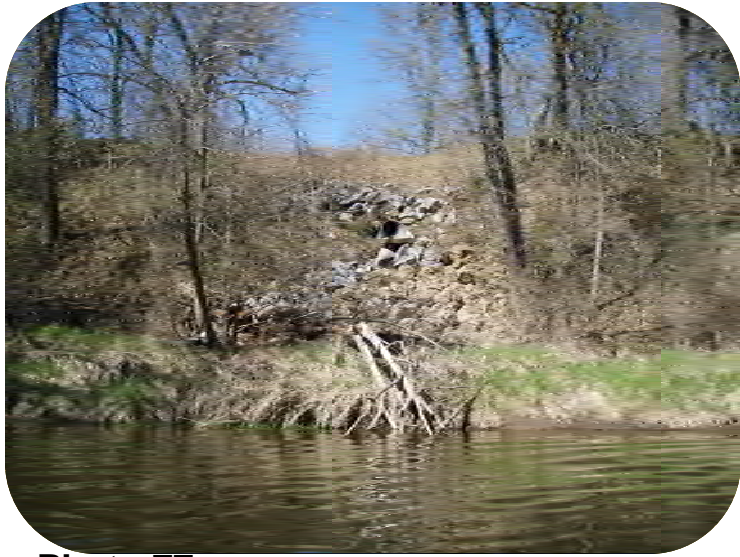
Photo 77 – Approx. 18 in. outlet at midpoint of slope with flowing water, rock above and below, and no erosion.
