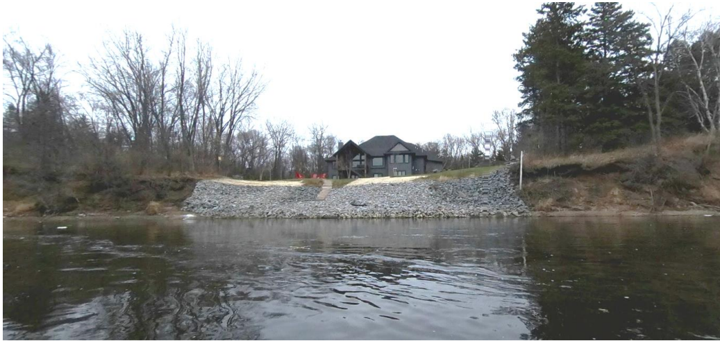
Figure 3. Riverbank stabilized with riprap bordered on both sides by severely failing vertical slopes.
