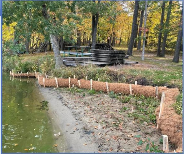
Biolog installation. October 2022.
